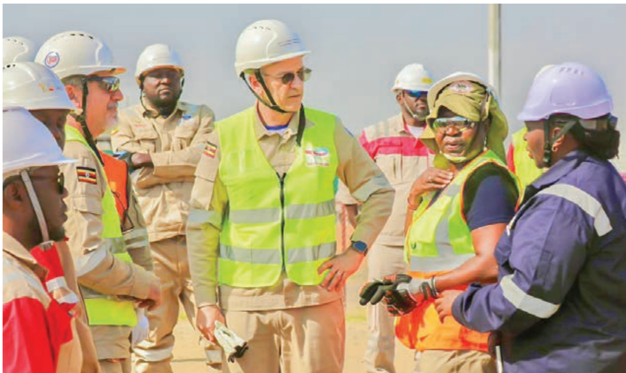
Hon. Nankabirwa inspecting progress of the Albertine project in preparation for first oil. Next to her is Permanent Secretary Eng. Irene Bateebe
